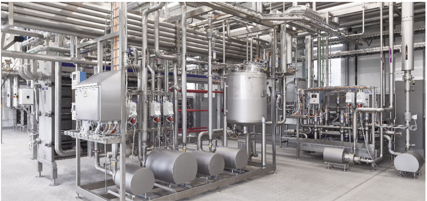
The central plant area with tubular heat exchanger
