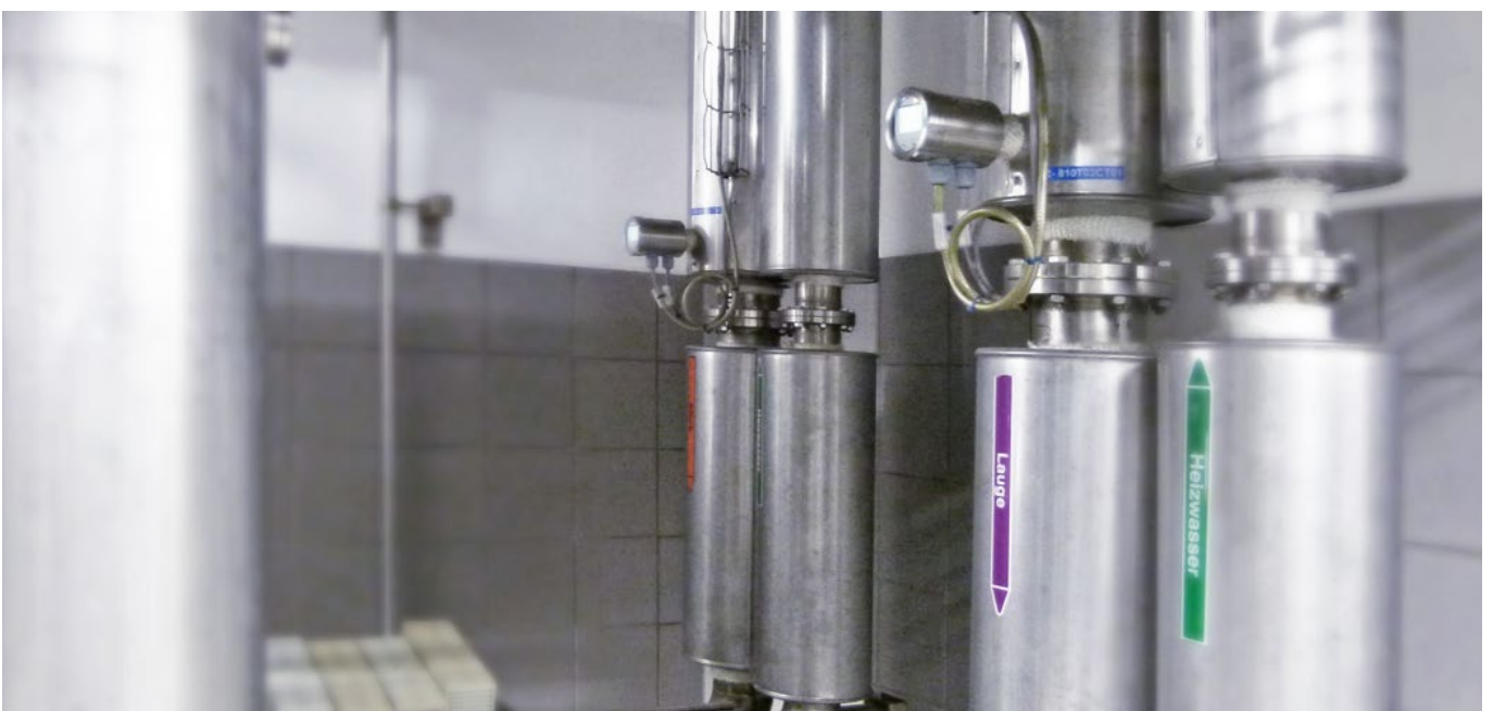
ILM-4 in the CIP feed and return flow
